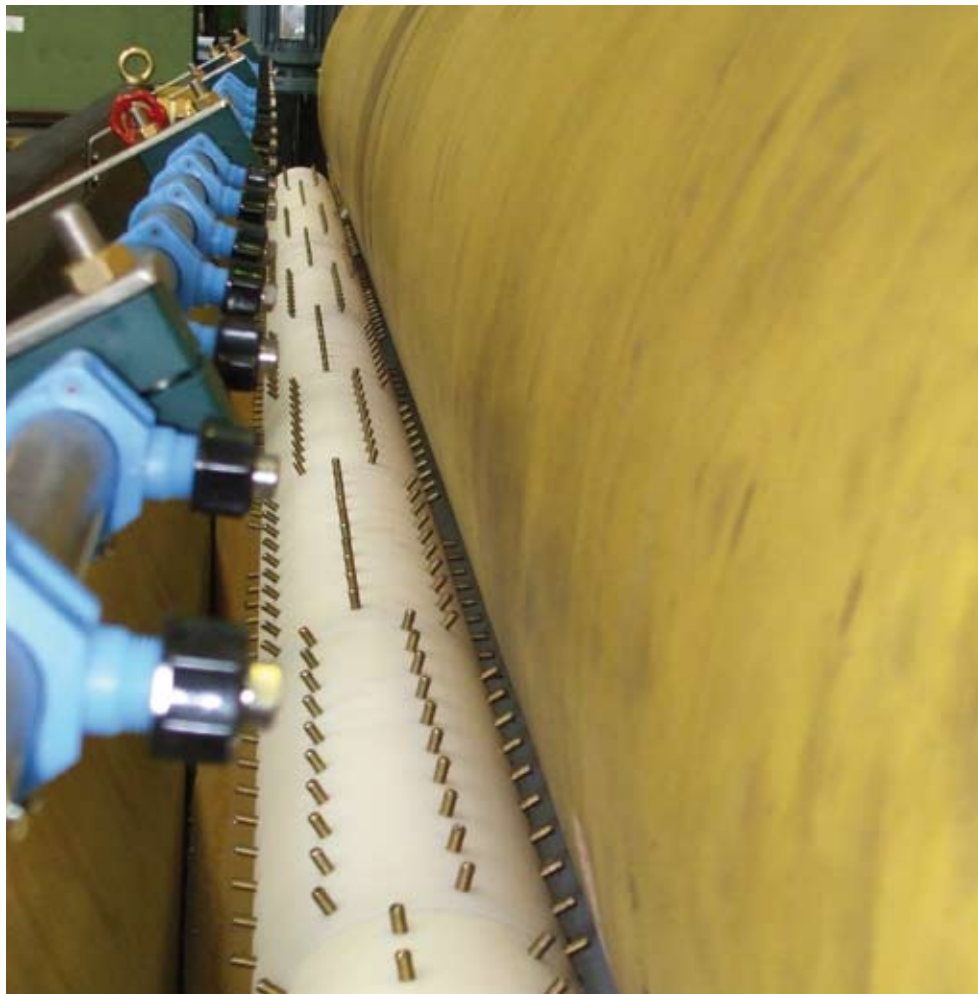
Discharge roll and wash water spray
